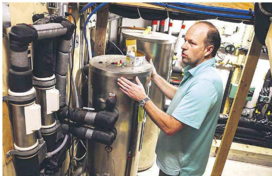
Rob Steels with the insulated water tanks in the mechanical room in his house, which is heated and cooled by a geothermal system and also has 2-foot-deep insulated walls.
